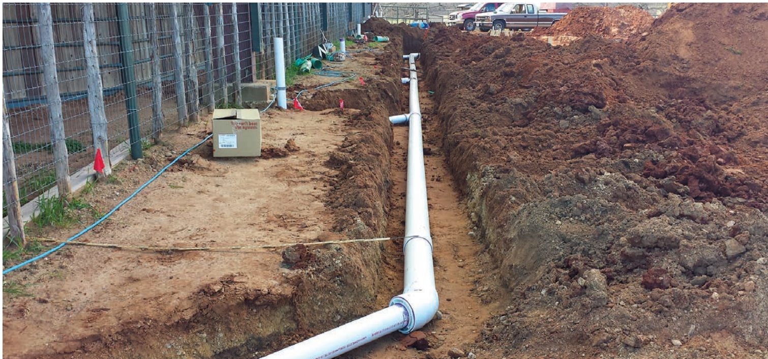
A “wet system” routes rainwater through underground pipes to collection tanks. Some systems that collect rainwater can even be used to make water drinkable; however, homeowners should check with local and state water boards to ensure laws do not prohibit rainwater collection.
