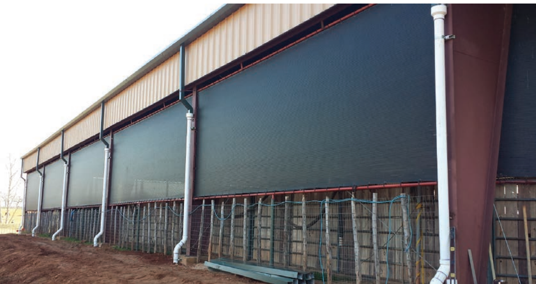
Circle Y's 28,000-square-foot arena roof allows for approximately 16,800 gallons of water collection per inch of rain.
