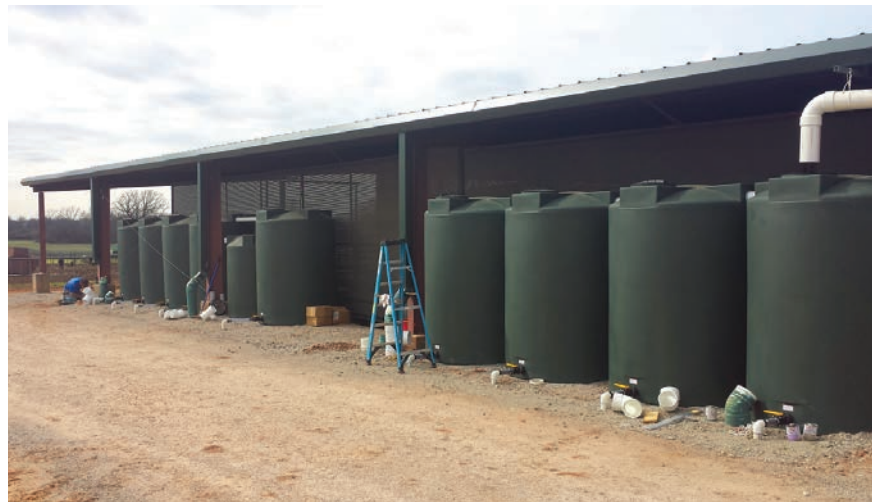
Nine, 1,150-gallon tanks were installed on the south side of the Circle Y arena, where they were able to be tucked out of the way of the road.
