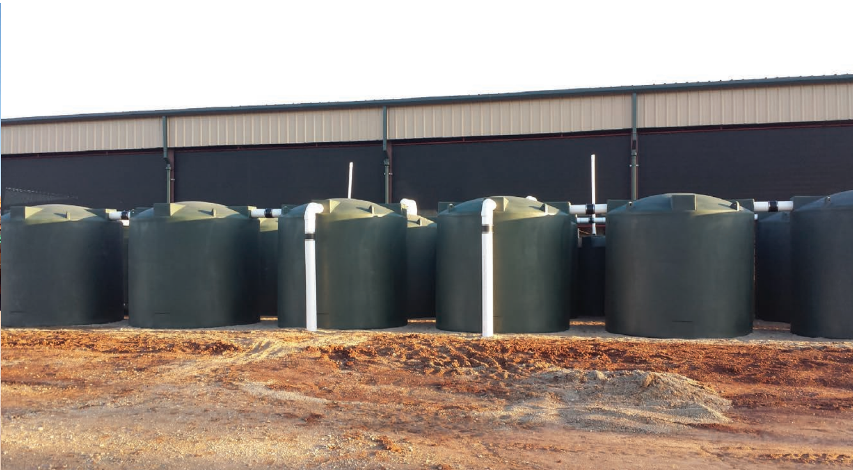
Rainwater collection, which has been used for centuries, is regaining popularity. The largest, most involved system at Circle Y consists of 12 2,500-gallon tanks that can be drawn from at a single source. The PVC collection piping replaces the metal gutters approximately 15-feet above ground level, and carries the collected rainwater underground to the tanks.
